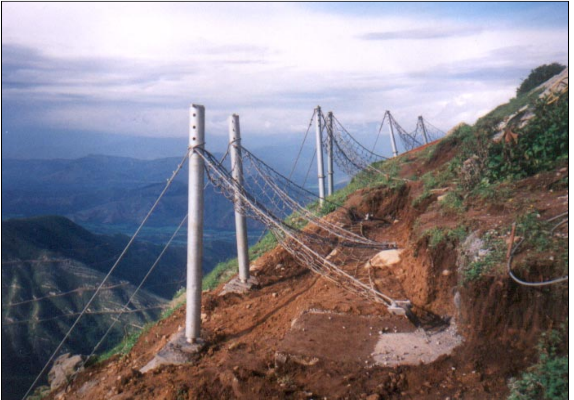
Avalanche Control Structures installed at an avalanche site on NH-1A (Jammu-Srinagar Highway)
